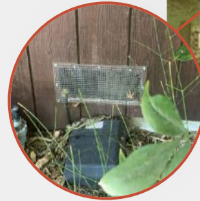
Vent greater than 1/8" opening
