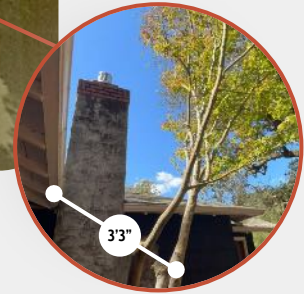
Tree within Zone 0, 10' of chimney, & overhanging roof
